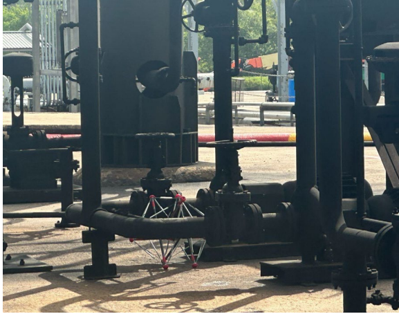
Fig. 15: 4-Gas PLUS sensor placed near potential leak site
