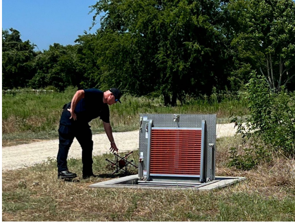
Fig. 25: 4-Gas PLUS sensor deployed at entrance of subterranean tunnel
